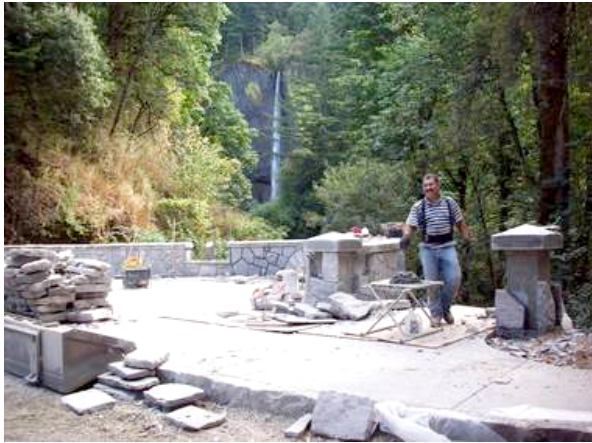
Doug Theil, a masonry worker for Nature's Edge Stone Art, Inc., works on walls at Latourell Falls that historically match the original retaining walls on the Historic Columbia River Highway completed in 1915.
